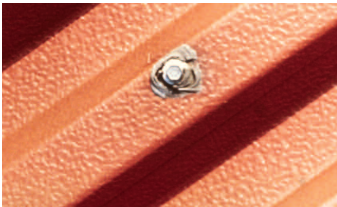
Damaged fastener on roof cladding.
