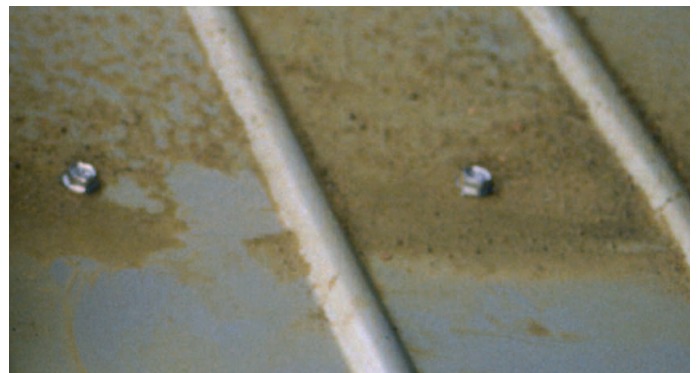
Mould growth on pre-finished steel cladding.
